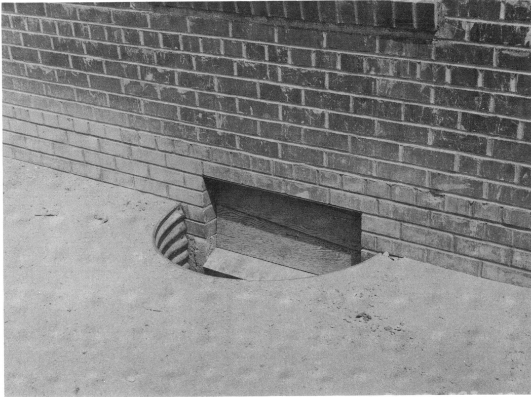
Fig. 2.21 — Basement window well before sandbagging.
